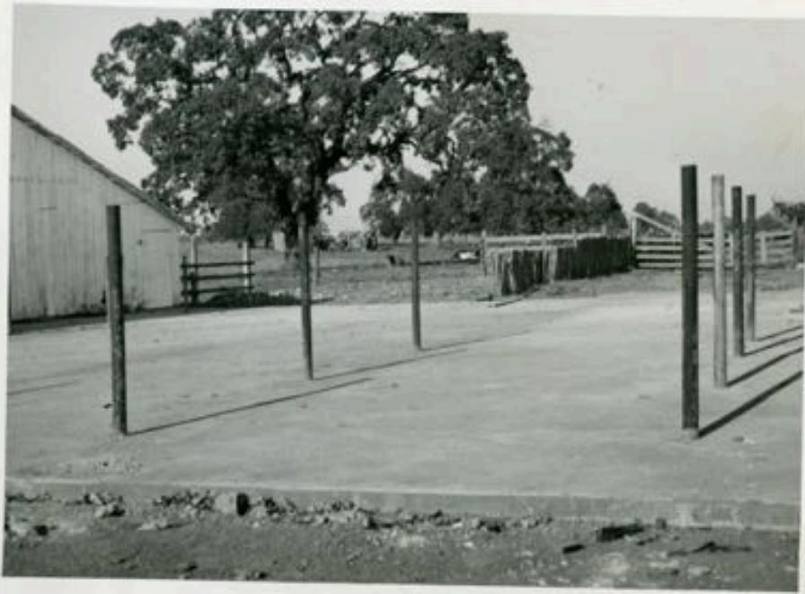
CONCRETE CORRALS AND RAMPS ARE THE KEY - NOTE TOWARD SANITATION DURING WINTER MONTHS
