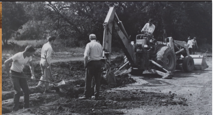
May 22, 1974—Dan Stewart on the backhoe and Bob Manzoni in the trenches
