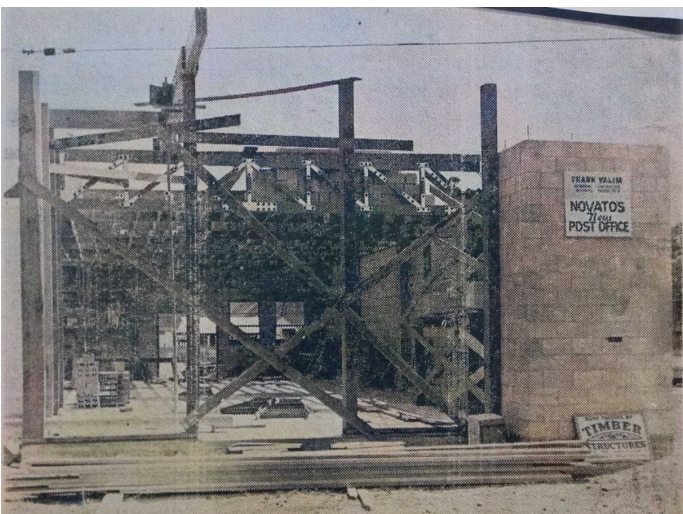
New Post office being built on the corner of Machin and Vallejo. Sign says "Frank Valim General Contractor Novato New Post Office" Novato Advance - September 28, 1951
