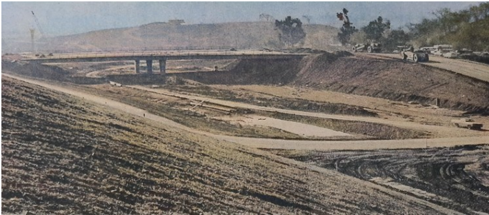
“Pictured here is the New DeLong Avenue overpass. Work on the Novato freeway bypass project has been moving along at a slow, and not particularly steady, pace during the past few months because of some of the worst weather in the city's history.”
