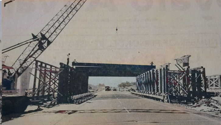
Lew Jones Construction Company finally put a top on the new Rowland Avenue overpass on Highway 101.
